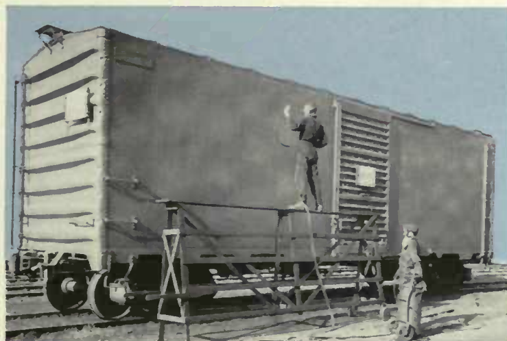
Painting a new freight car made of USS Cor-Ten, a weight-saving steel developed by U. S. Steel research.
